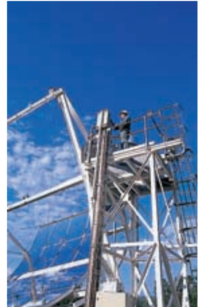
SCL HAS COMMITTED TO RESEARCH AND DEVELOPMENT OF SOLAR THERMAL TECHNOLOGY. HERE ANDREW EVANS - ELECTRICAL TECHNICIAN ADJUSTS SOLAR MIRROR ALIGNMENT OF THE DEMONSTRATION SOLAR CONCENTRATOR AT STANWELL POWER STATION.
