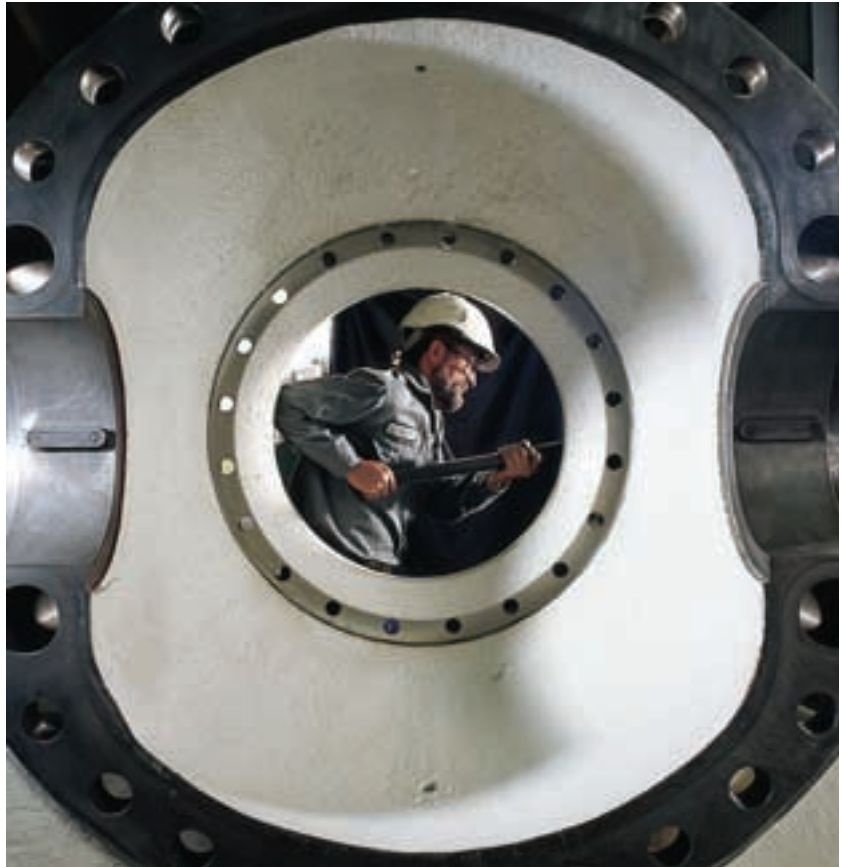
RHODNEY DODDS - FITTER REASSEMBLES A STRAIGHT FLOW VALVE AFTER RECONDITIONING, PART OF THE KAREEYA HYDRO HALF-LIFE REFIT.
