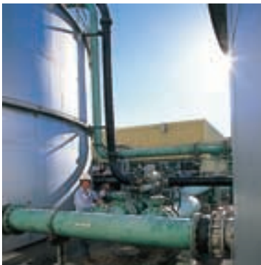
DAVE MILLICAN - CHEMICAL PLANT TECHNICIAN INSPECTS VALVES AT STANWELL POWER STATION'S WATER TREATMENT PLANT, AS PART OF A ROUTINE MAINTENANCE PROGRAM.
