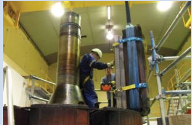
The one metre long wedge keys being removed from one of the 10 rotor poles.
